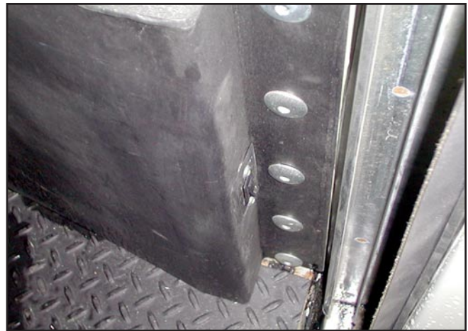
Illustration DE-5 Switch and Hucktainer Fasteners on a Deflector Plate
