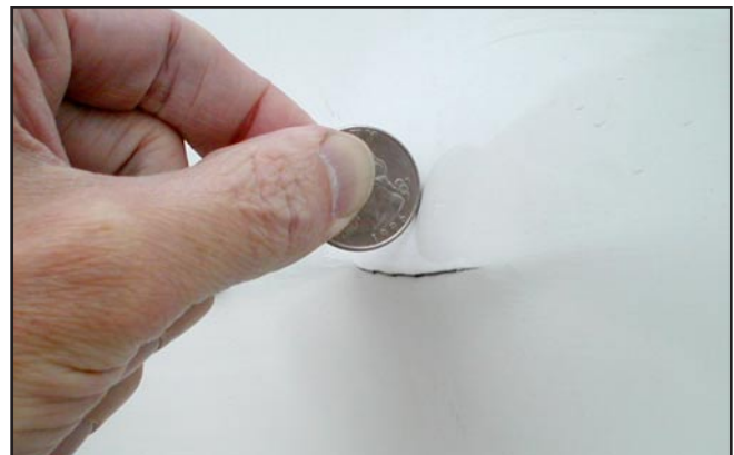
Illustration PL-5 Tap Across Damaged Area to Test for Delamination
